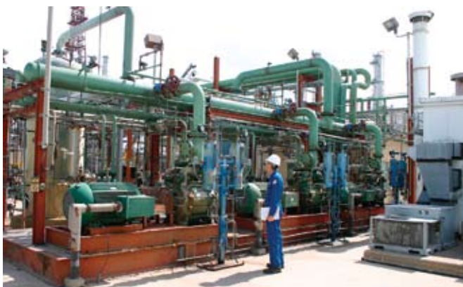
FIG. 4 An FGRU at the FHR West Plant in Corpus Christi, Texas.
