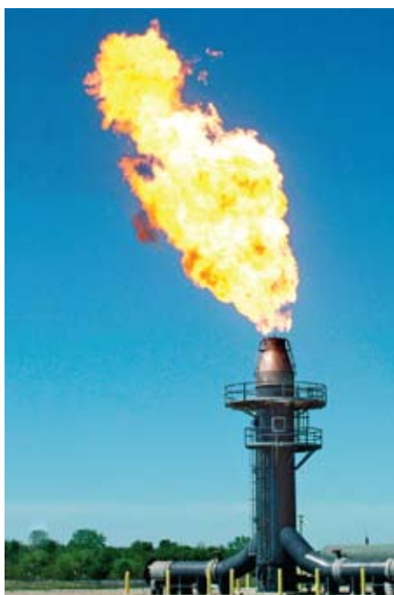
FIG. 1 Example of an air-assisted flare during testing.
